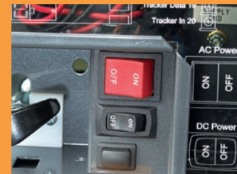
Built-in AC and DC power switch
